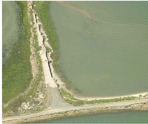
Chula Vista Wildlife Island levee erosion
